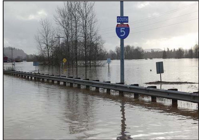
I-5 Southbound completely submerged
